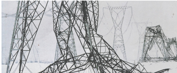
Figure 1. High voltage transmission towers damaged due to an ice storm in North America, January 1998. Picture reproduced from [5].
